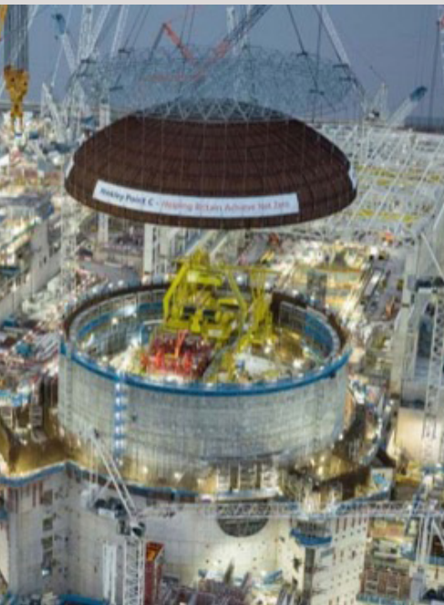
The 245-tonne domed roof being placed on the first reactor building in December 2023. Photo credit: EDF
